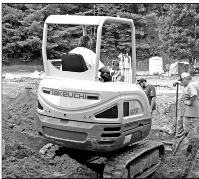
Construction is underway to build 10 new classrooms at Union County Primary School. Photo/Shawn Jarrard
