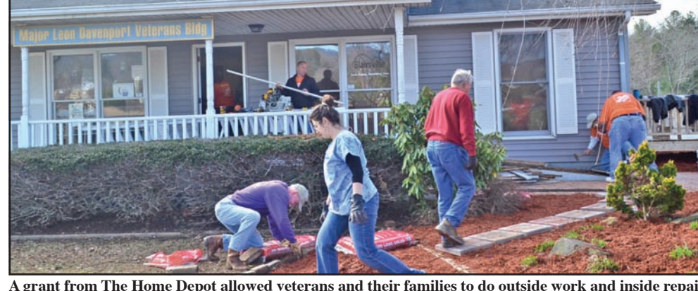
A grant from The Home Depot allowed veterans and their families to do outside work and inside repairs at the Major Leon Davenport Veterans Building off Georgia 515 in Blairsville. Photo/Lowell Nicholson
